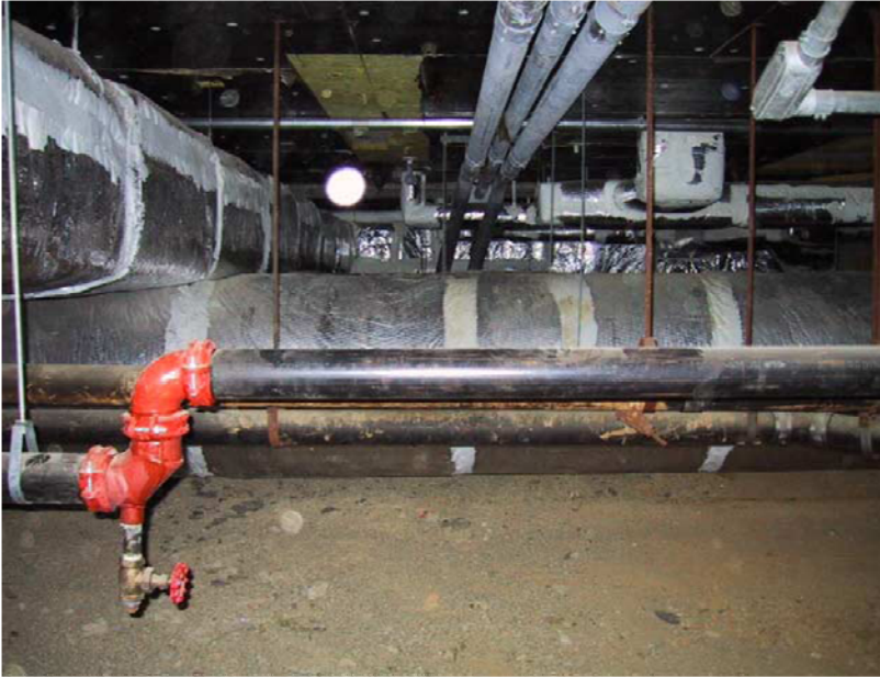
Figure 3.9 Lack of Mechanical Crawl Space Constrained Conversion
