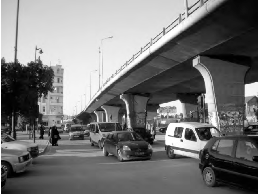
Figure 5.4. Avenue de la République/Z4 viaduct over the Avenue Bourguiba, Tunis. Photograph (2009). (Source: Author's collection.)
