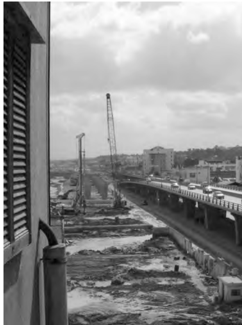
Figure 6.2. Construction of the Z4 extension north of the Avenue Bourguiba, Tunis. Photograph (2009). (Source: Author's collection.)
