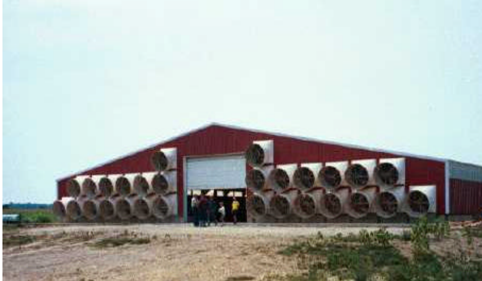
Figure 3. 60-Inch Tunnel Fans on a Six-Row Freestall Barn.
