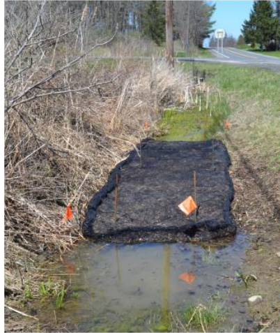
Figure 5-1: Ditch bioreactor right after installation. A cloth netting contained the woodchips and four rebar stakes secured the bioreactor during high flow rates and helped maintain its shape.
