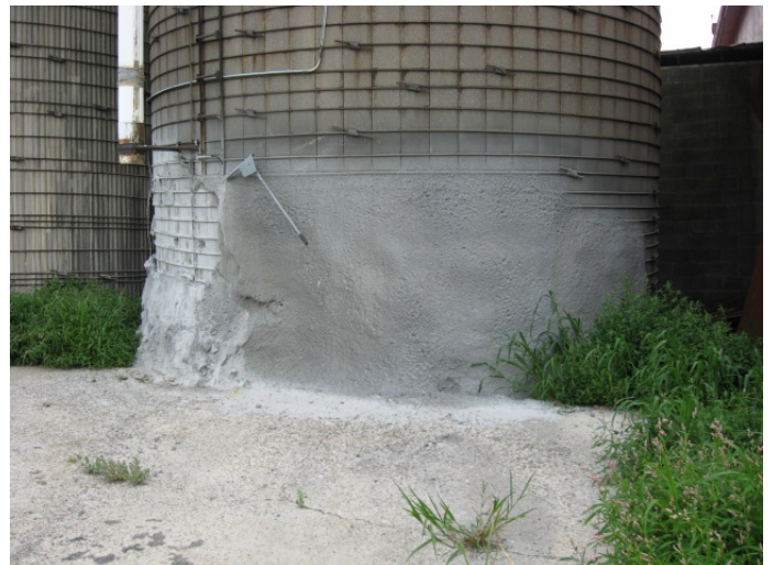
Base of silo temporarily reinforced with "shotcrete" concrete. Photo taken July 2008, used with permission of owner. The silo will be taken down this fall.
