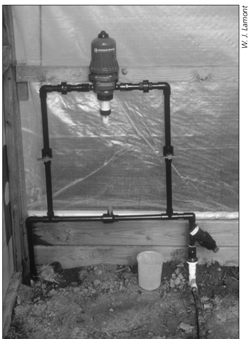
Photo 3-18. Water-powered Dosatron injector pump.
