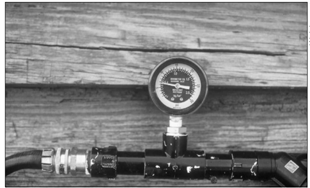
Photo 3-15. Pressure gauge for a small system showing 7–8 pounds of pressure.
