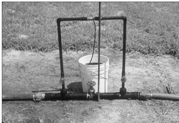
Photo 1-7. Small venturi unit used for fertigation.
