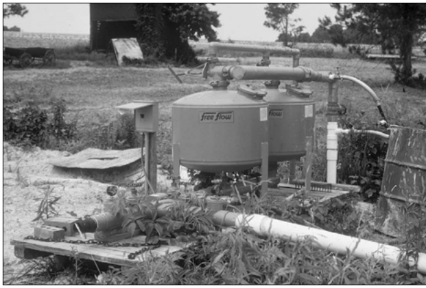
Photo 3-14. Large 4-foot-diameter sand media filter.
