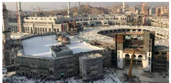
Figure 12. Renovation and expansion work in the Masjid Al-Haram in Mecca (Photo Credit: Ali Daye).
