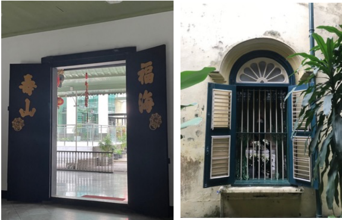
Figure 3.37. Two-leafed Solid Wooden Door at Candra Naya (left) and Figure 3.38. Window Shutters over Cast Iron Grills at the Tjong A Fie Mansion (right) (Source: The Author's Collection)
