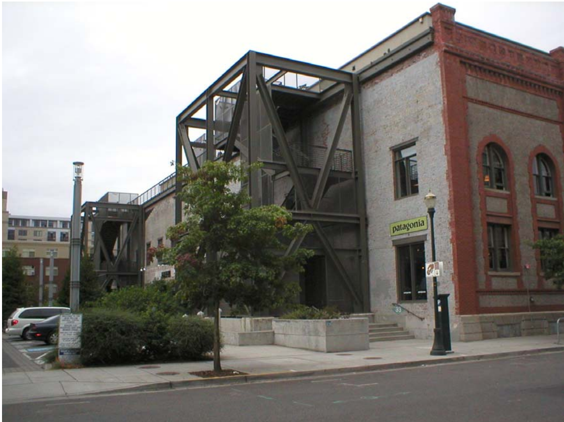
Figure 5.9 - Steel tower seismic code upgrades (Photo credit: Author)
