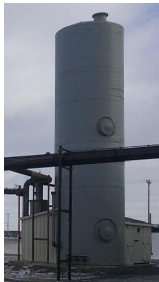
Figure 1. Sunnyside biological trickling filter
