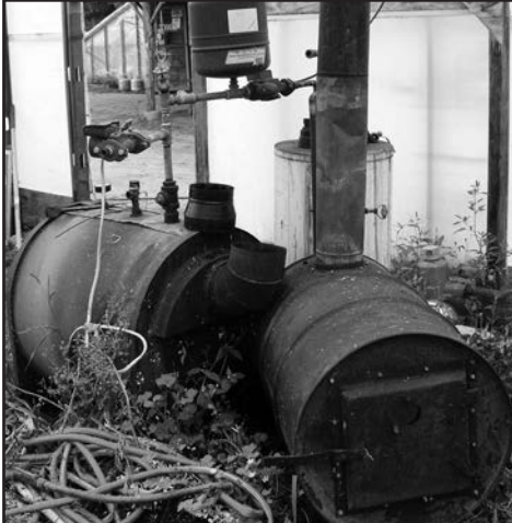
Grindstone's wood-fired boiler.
