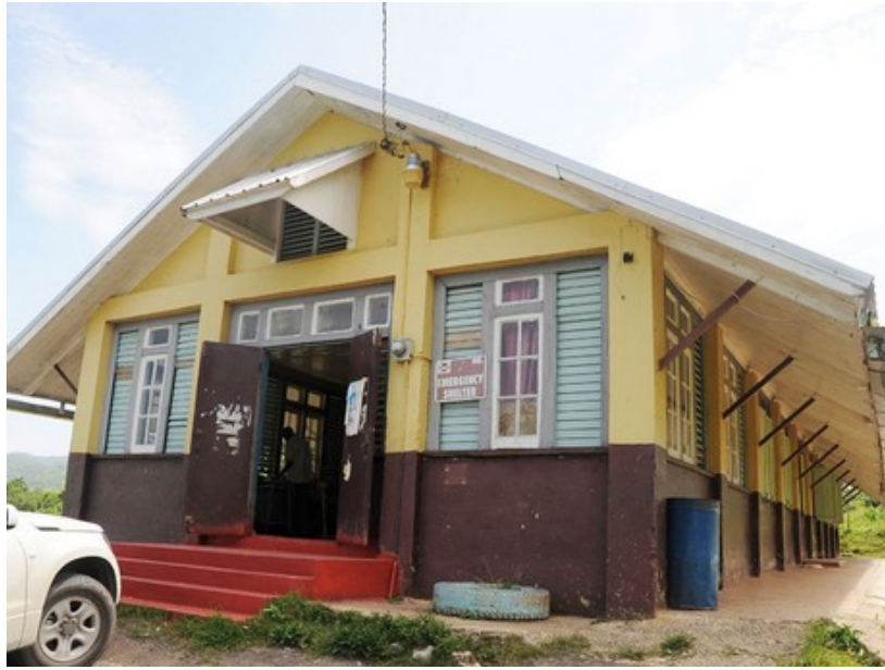
Figure 6. Assessment of the external façade - included windows, doors, steps, walkways, wall surfaces, eaves, lighting and signage. Photo adapted from “Primary school needs facelift” by Christopher Thomas. Retrieved from http://jamaica-gleaner.com/gleaner/20110813/news/news9.html
