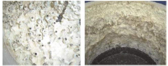
Figure 2. Accumulation of elemental sulfur on the digester walls and cover when netting is not used. 5
