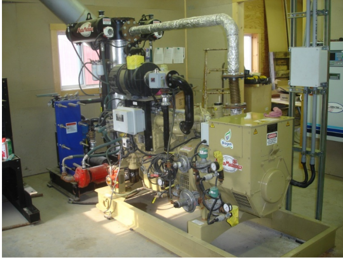
Figure 26. Wagner Farm EGS with heat recovery system (Source: Gooch, 2009).
