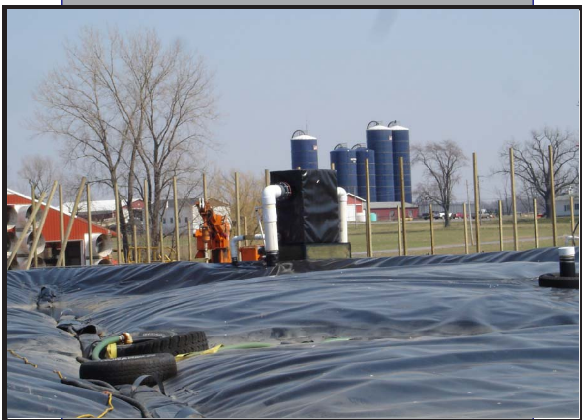
Patterson Farms Complete mix digester
