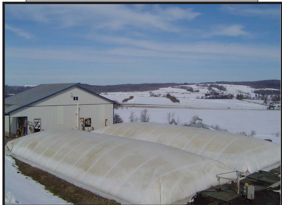
Ridgeline Dairy Horizontal complete mix digester (soft top)
