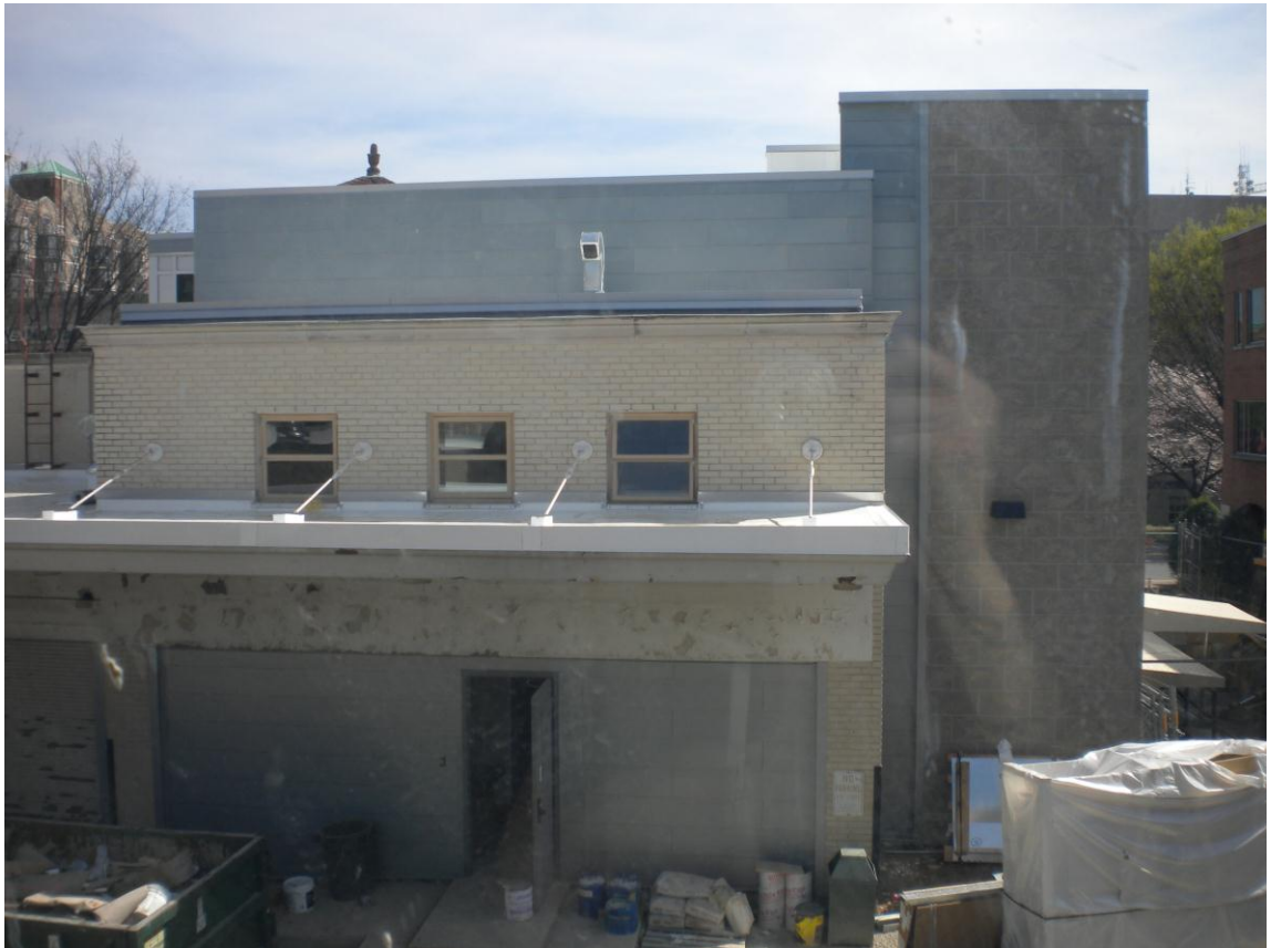
Illustration 17: New Roof Monitor and Elevator Shaft. (Source: Personal photograph by author. 3 Mar. 2012)
