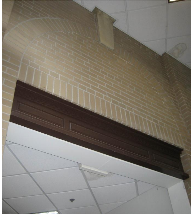
Illustration 9: Opening Created by Removal of Window. (Source: Personal photograph by author. 25 July 2012)
