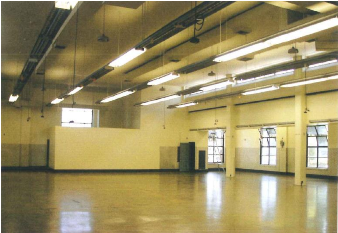
Illustration 22: Photograph of Workroom Prior to Rehabilitation. (Source: Jeffrey Chusid. Beverly Hills Post Office Preservation Study . Sept. 2001)
