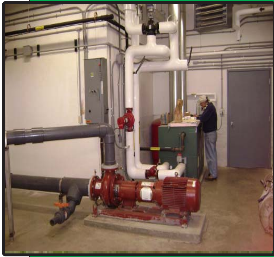
Roto Mix system - 30HP Mixing pump
