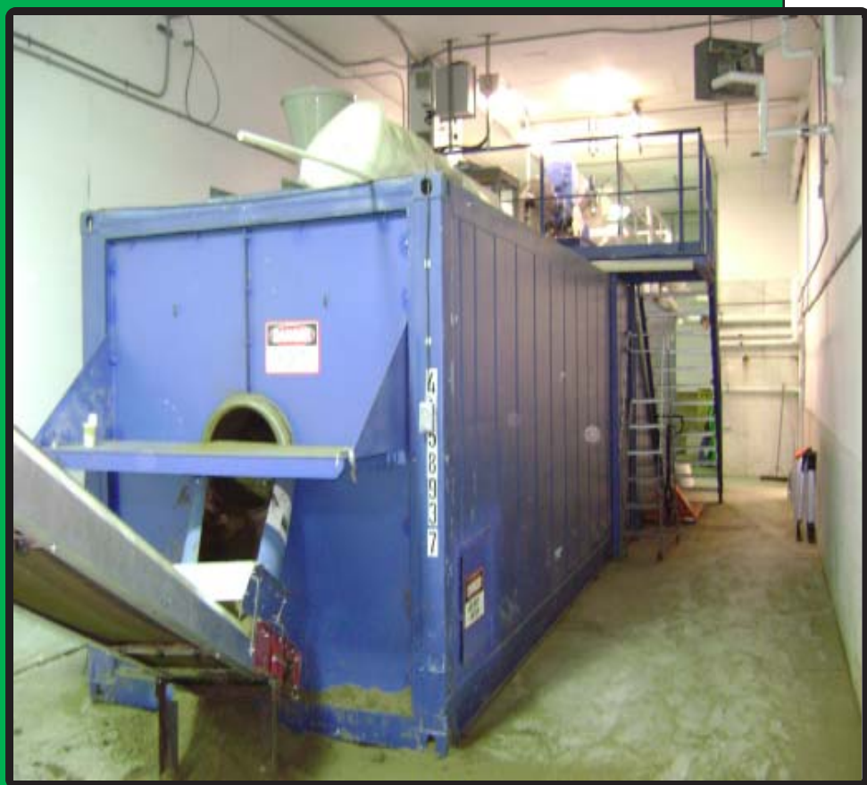
Bedding Recovery Unit. The farm separates influent prior to digestions to make solids for bedding.
