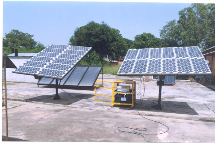
Plate 1. Arrangement and connections of solar photovoltaic panel, energy storage (batteries) and power conditioning system.
