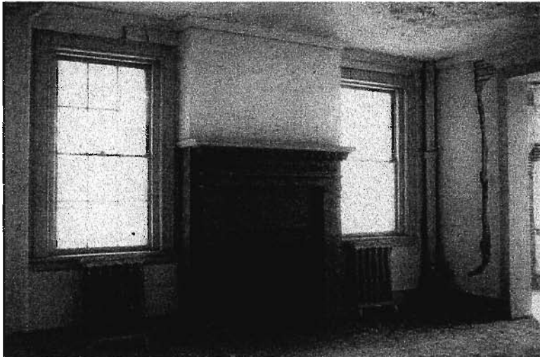
Figure 7: View of Room 103, east side of main block, showing 6/6 windows on either side of brick fireplace.
