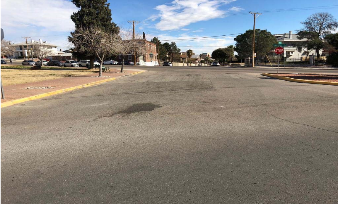
Figure D-1. Buffer or road separation missing on Upson Dr.
