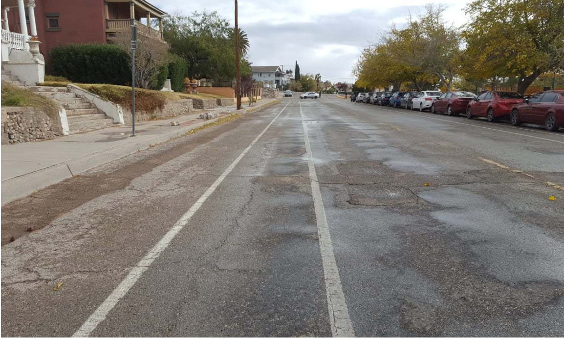
Fig A-5. Fair Illumination rating since lighting exists but is limited on Prospect St.
