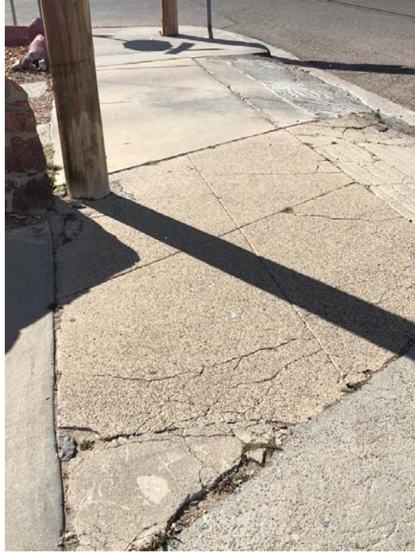
Figure B-3. Localized deteriorated sidewalk with cracks on Yandell Dr.
