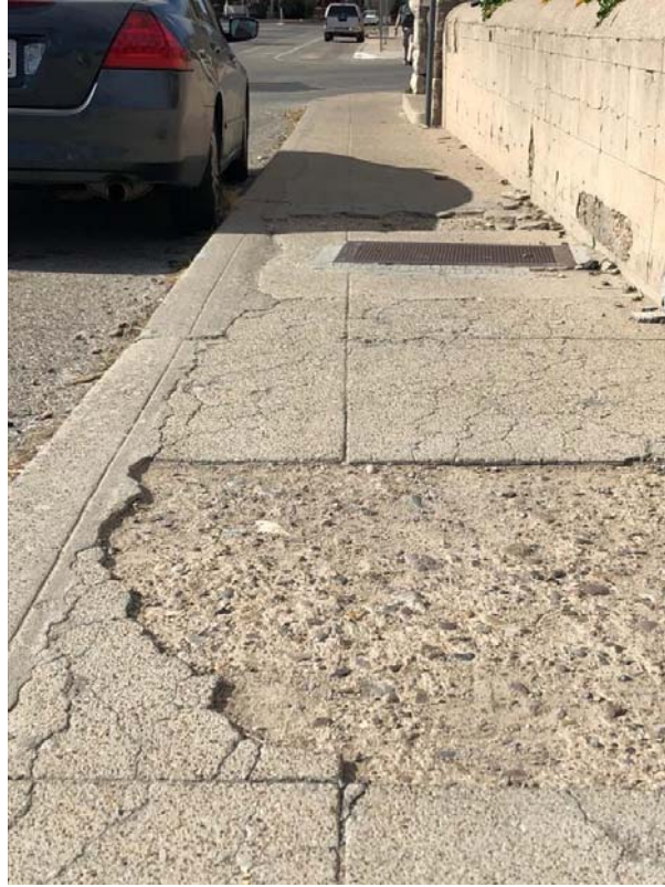
Figure A-3. Localized minor cracking and raveling on the sidewalk of Prospect St.
