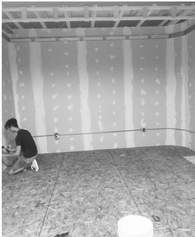
Figure 3: A photo of the build-out at Inclusive Recording in-progress. Courtesy of Inclusive Recording (2016).
