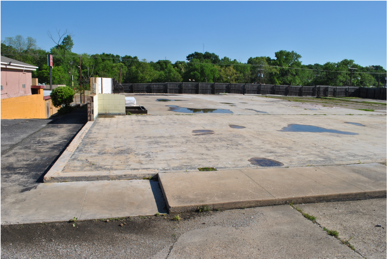
Illustration 8.12. Foundation near the entrance at the American Inn in Tyler. Photo by Author.
