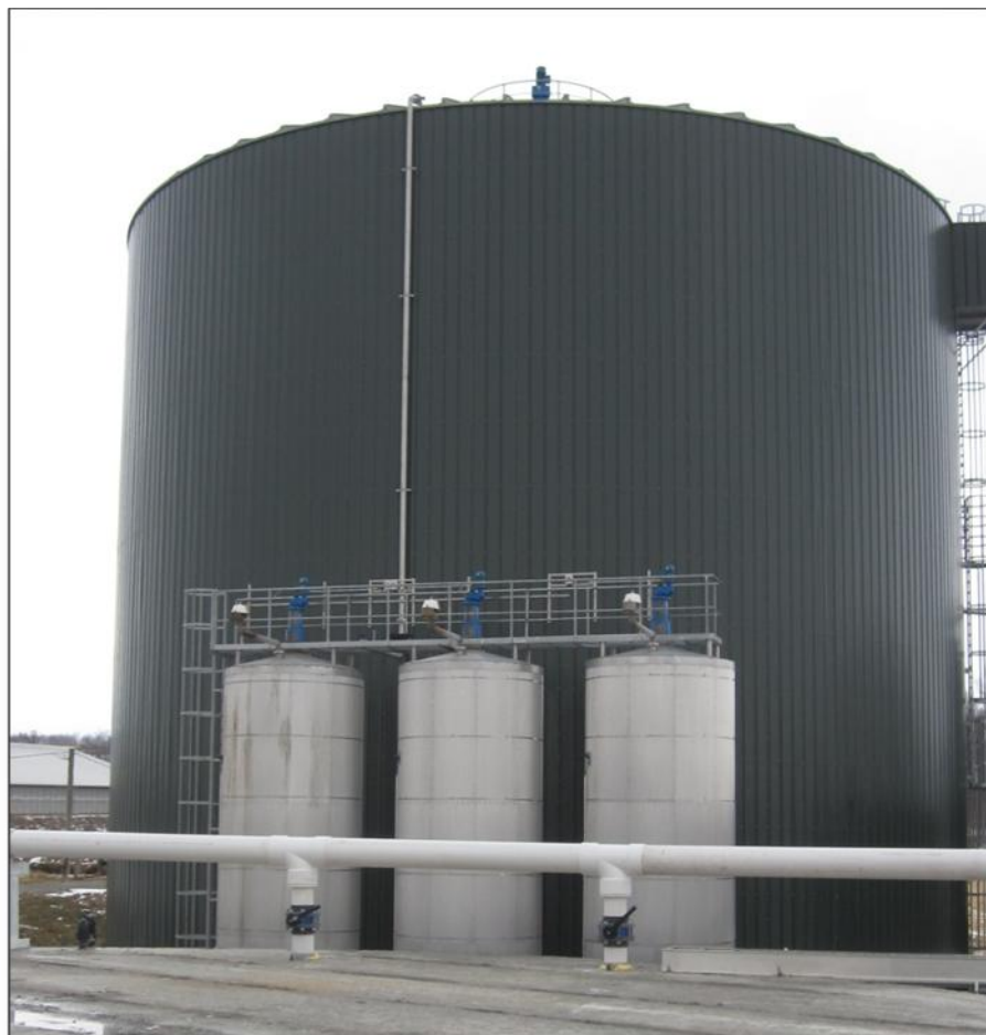
Figure 3. Continuously-stirred tank reactor and pasteurization units
