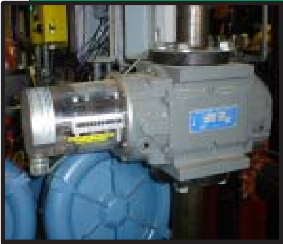
A ROOTS gas flow meter measures the flow of biogas to the engine-generator set
