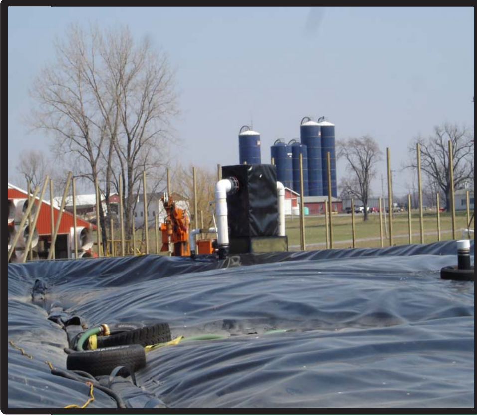
View of digester cover
