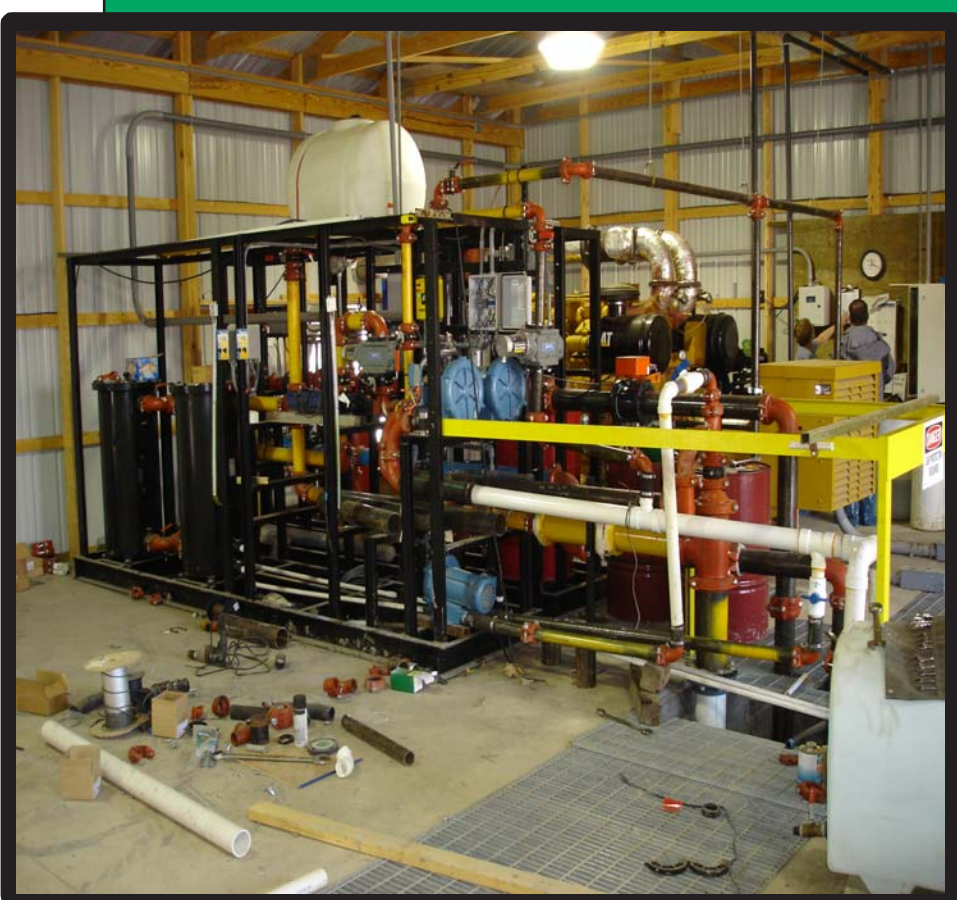
Engine-generator set in gas utilization building
