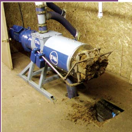
Solids separation necessary for low solids content digestion
