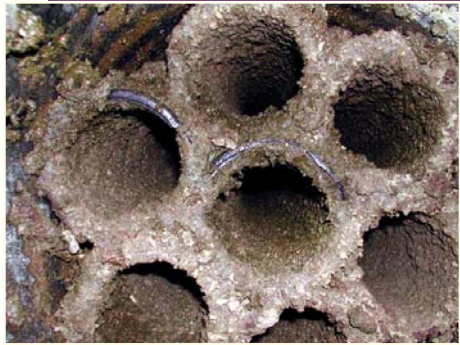
Fixed Film plugged with \text{CaCO}_3 sediment
