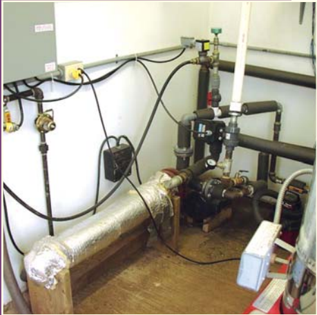
Back flush system installed to reduce heat exchange plugging.
