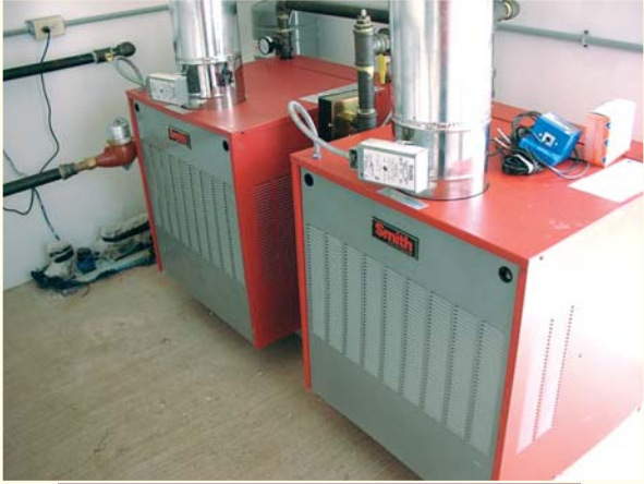
Propane (start-up) and Biogas (main) boilers to maintain digester at 100°F.
