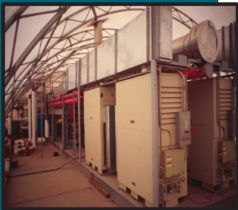
Microturbines in foreground and heating system in background
