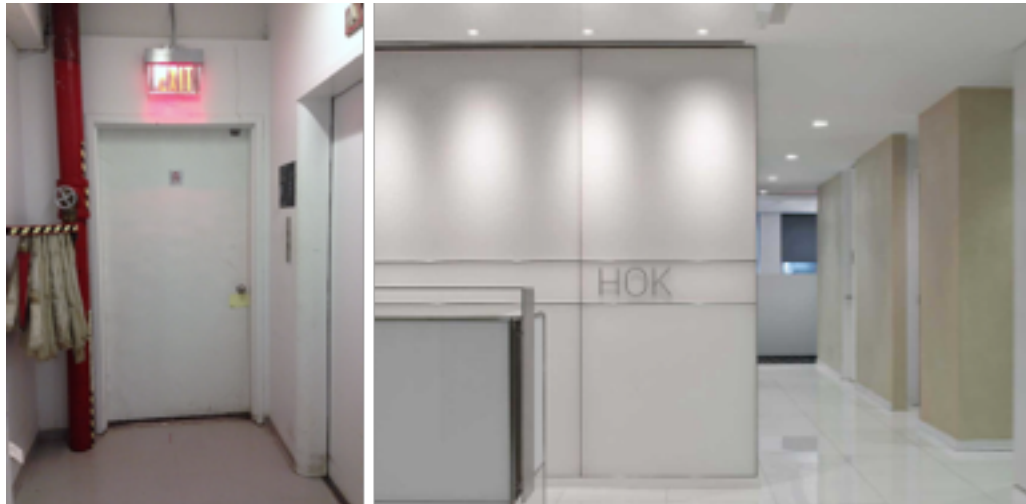
Image 4. Inaccessible Emergency Staircase Adjacent to the Reception Area
