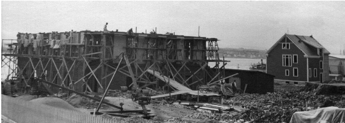
Figure 5.3. A photograph taken on October 8 th , 1913 showing the construction of the Bay Roberts Cable Building. From the Road to Yesterday Virtual Museum Exhibit.
