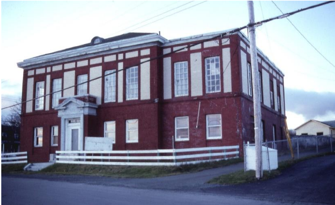
Figure 5.7. A 1994 photograph of the exterior of the cable building. Broken windows and falling bricks were major issues needing repair. From the Road to Yesterday Virtual Museum Exhibit.
