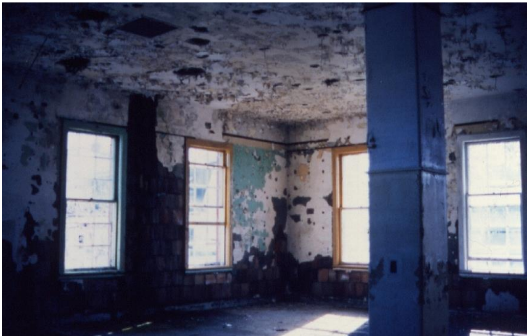
Figure 5.8. A 1994 photograph showing the interior of the former cable operations room. Mold was one of the biggest issues facing the restoration team. From the Road to Yesterday Virtual Museum Exhibit.
