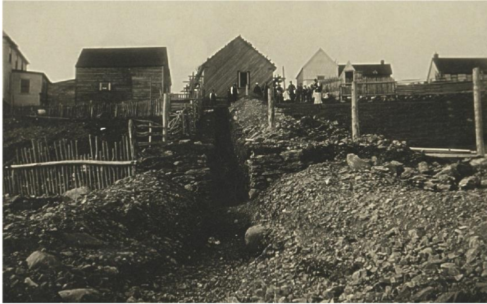
Figure 5.1. The cable trench leading from the shoreline to the first cable hut, July 22 nd , 1910. From the Road to Yesterday Virtual Museum Exhibit.
