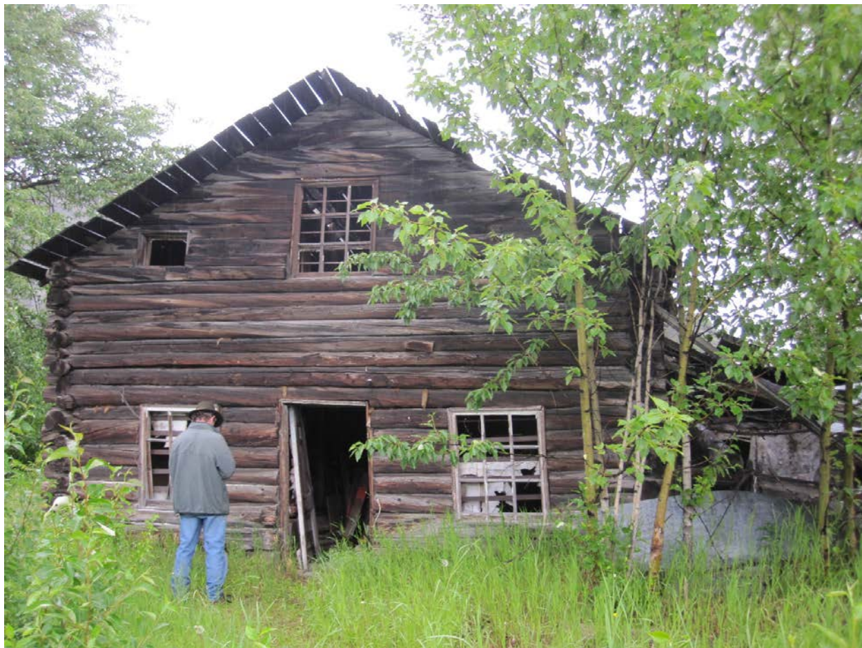
Figure 30. 1905 roadhouse at Gakona, standing to the side of the Gakona complex. Photo by Casey Woster.
