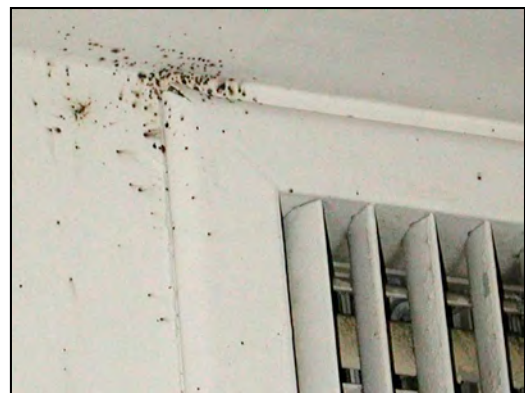
Bed bug fecal stains near a duct indicate harborage and possible movement. Photo by R. Cooper.
