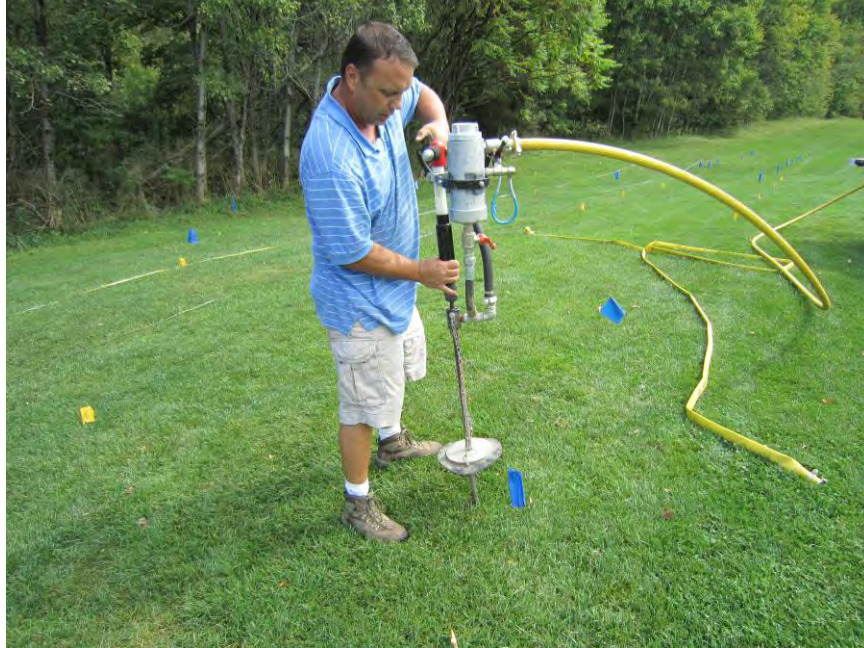
Figure 3 Cambridge Air Injection equipment
