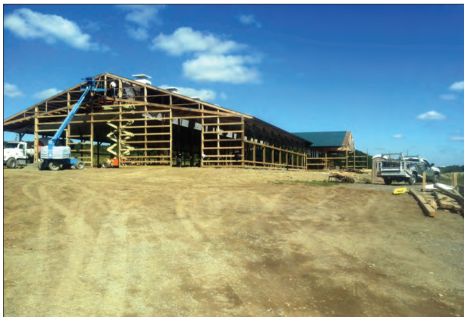
A Dairy Acceleration Project at Silver Meadows Farm included construction of a new barn. Photo credit: Russ Klein.
