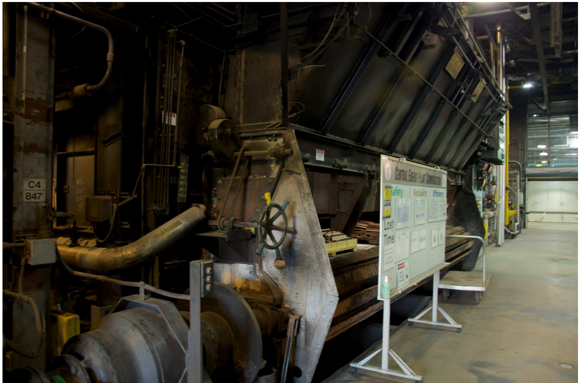
Figure 5: The mothballed Boiler #8, which has a hopper nearby which could be fed a solid fuel such as coal or biomass directly without any major conversions.
