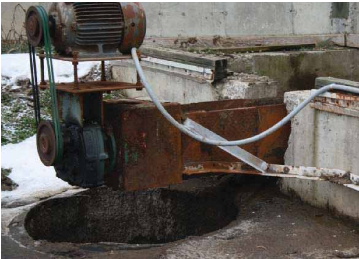
Photo 1. Auger depositing to a flush flume.
