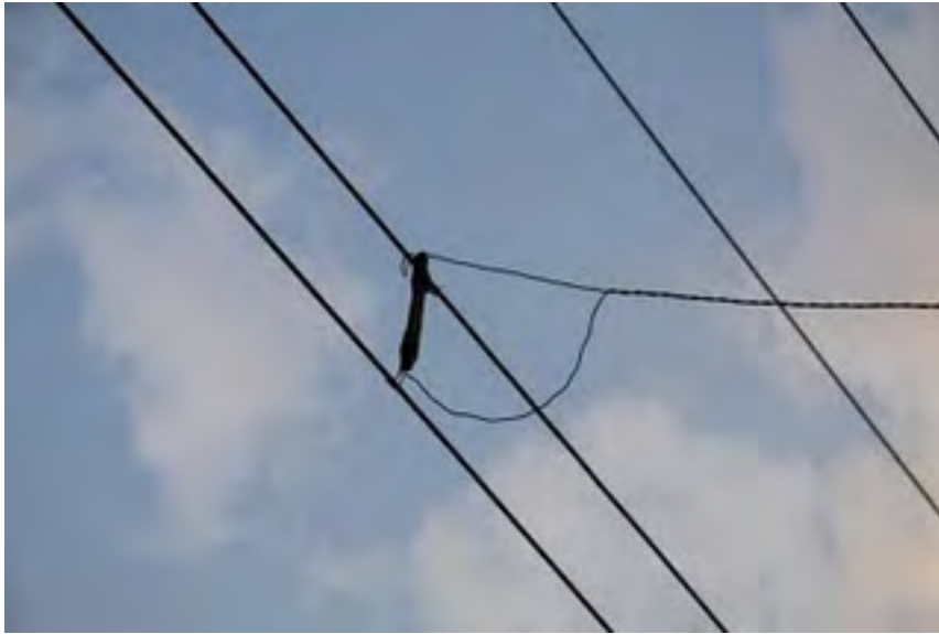
Figure 5.3: Illegal electrical hookup
