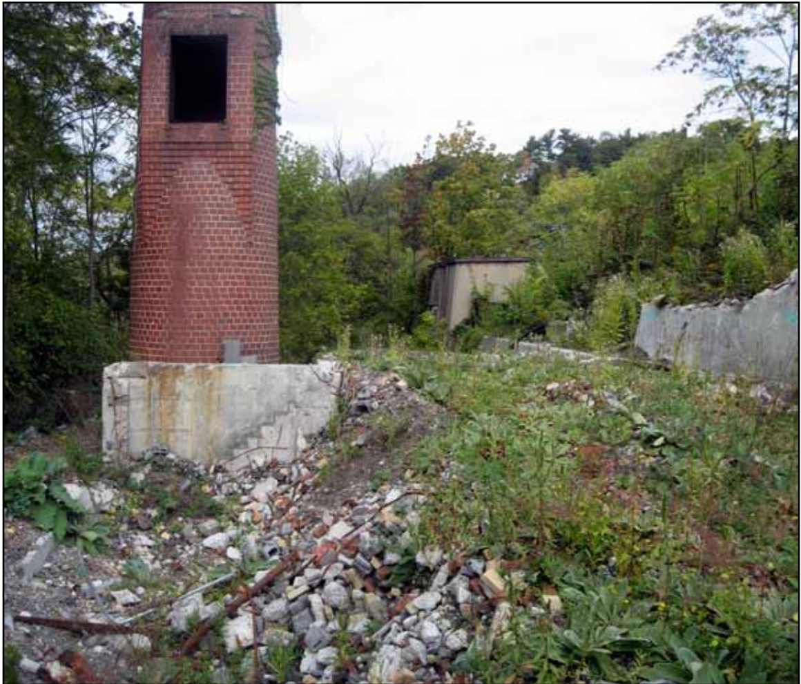
Fig. 91. Base of the smokestack with rubble from the demolition of the surrounding buildings. In the background is the last remaining building on the site. (Photograph by author).
