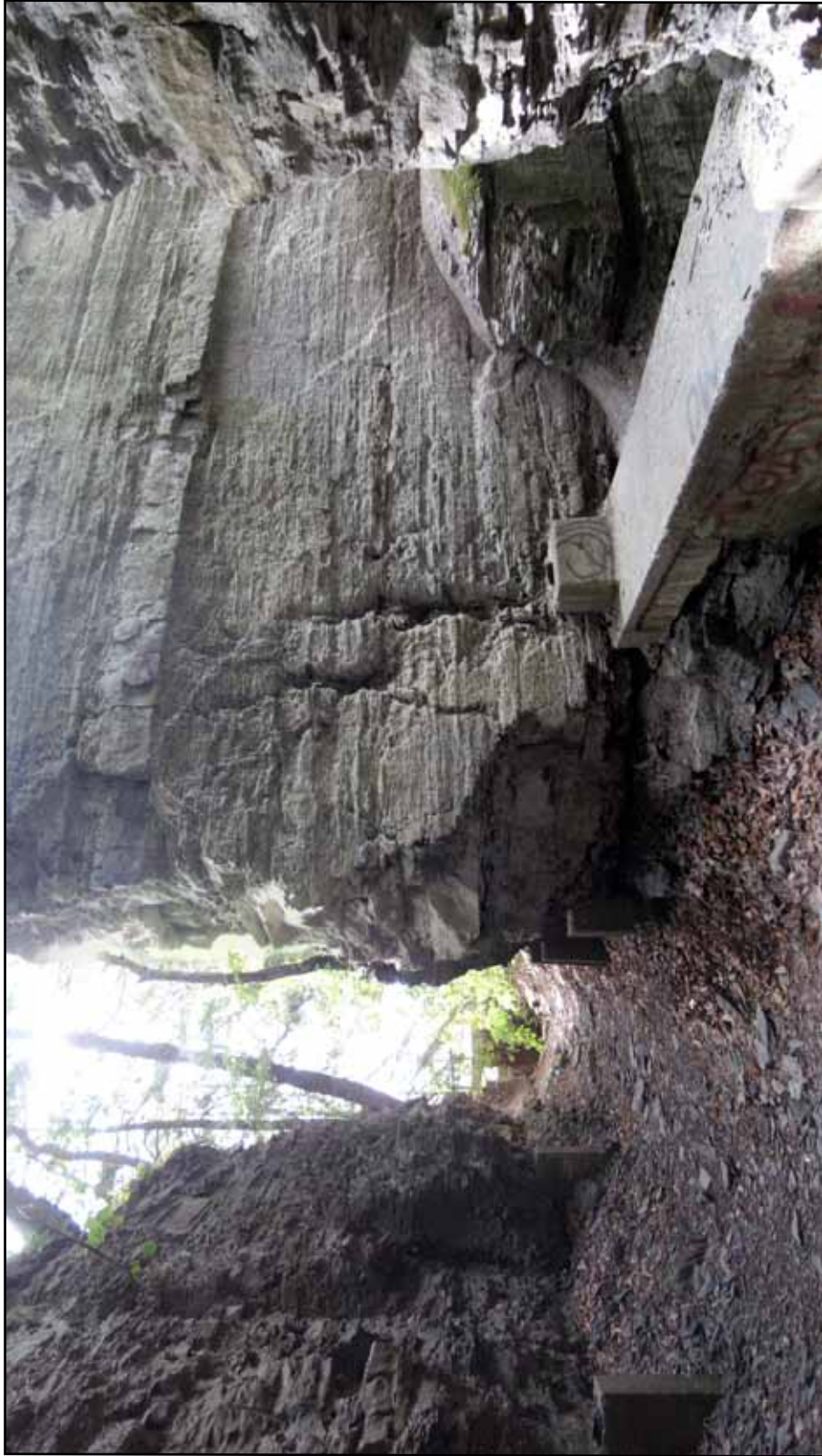
Fig. 105. Looking west down the raceway from the tunnel. At left is the lateral cut in the gorge that historically carried the wooden flume that first supplied the site's mills with water. In the background is the bulkhead that controlled water flow to the rest of the raceway. (Photograph by author).
