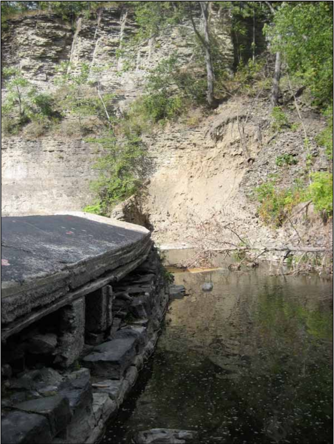
Fig. 99. Upstream side of the dam, where the concrete shell has deteriorated, showing the crumbling stone foundation and the opening of the spillway. (Photograph by author).
