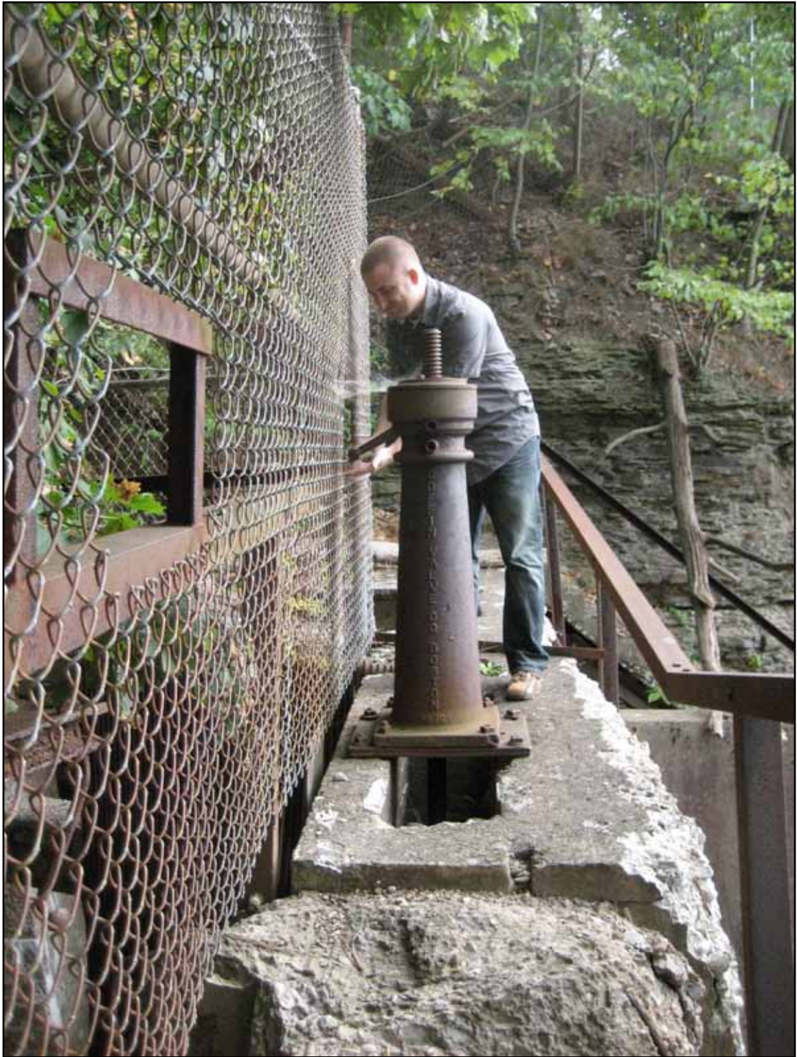
Fig. 107. Control mechanism at the top of the bulkhead. (Photograph by author).
