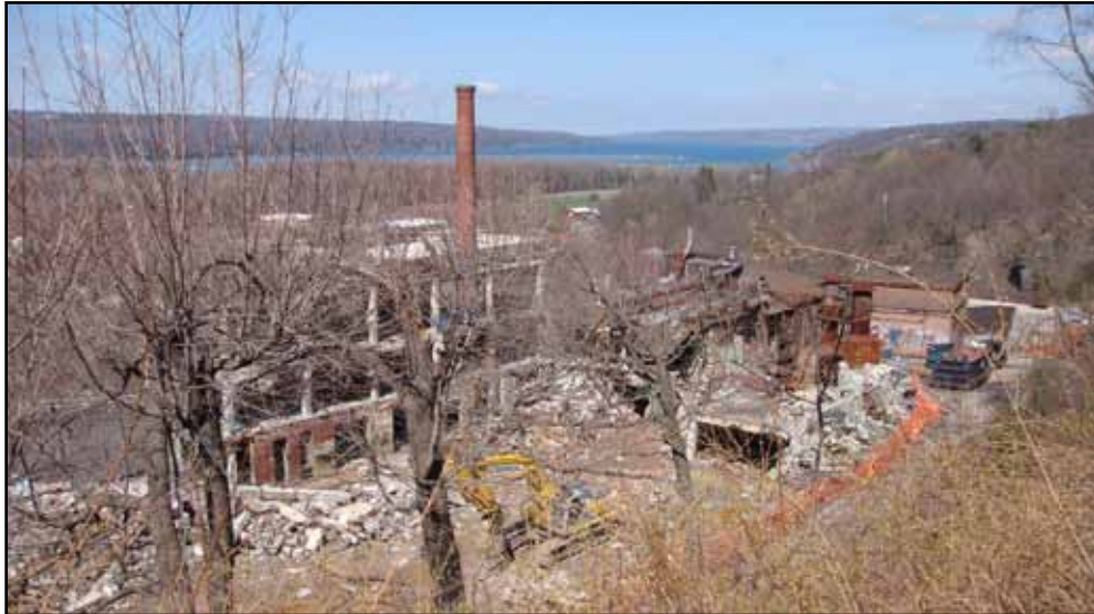
Fig. 61. View from slope above Gun Company of factory demolition. (Photograph by Leigh McGonagle, March 27, 2009).
