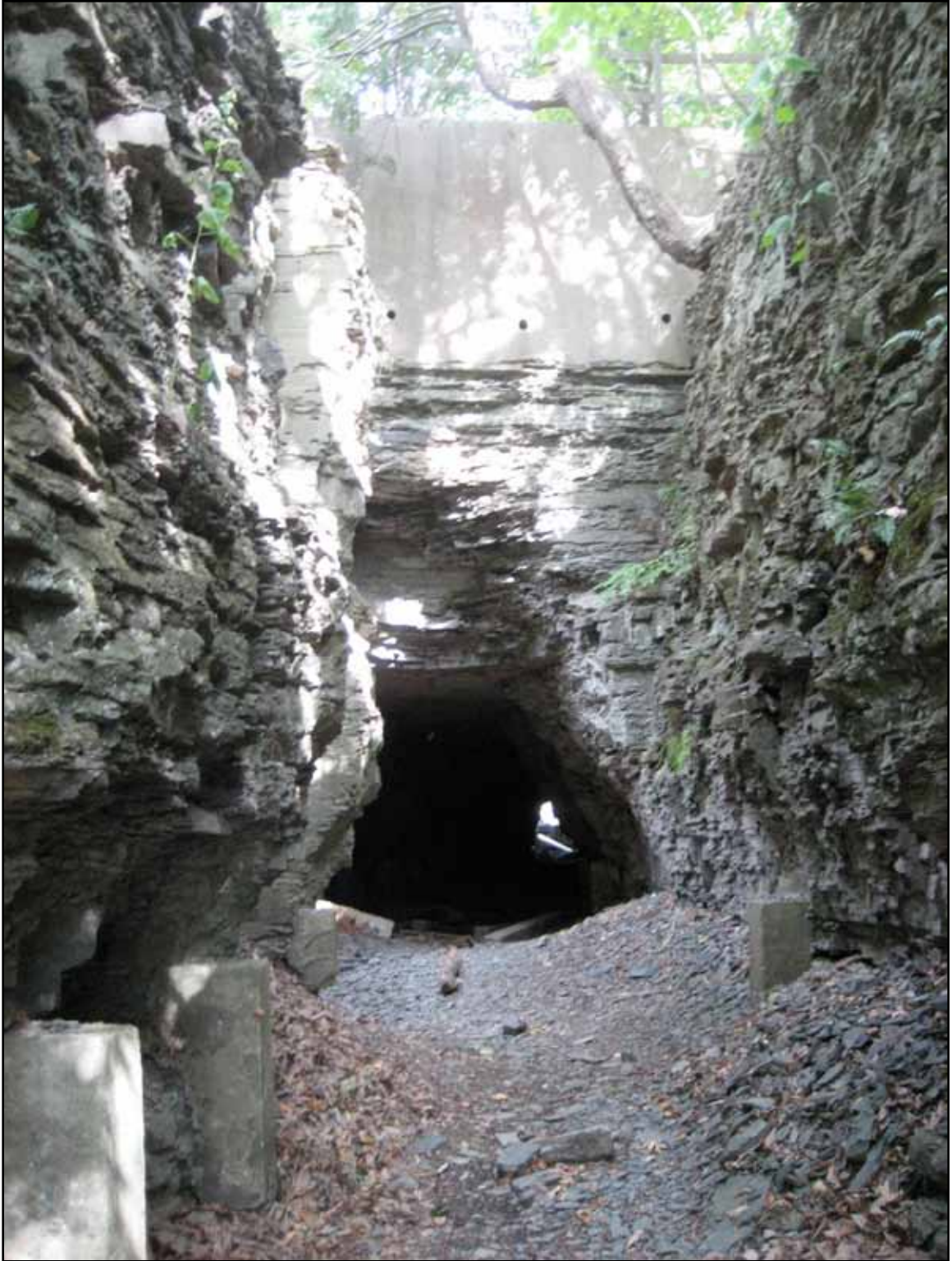
Fig. 104. The eastern mouth of the tunnel with supports for the wooden flume. (Photograph by author).
