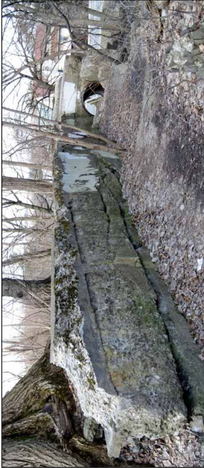
Fig. 115. Looking west along the flume that carried water from the end of the raceway to the Fall Creek Flour Mill, with the building's foundation in the background. (Photograph by author).
