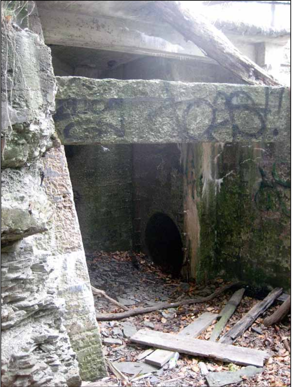
Fig. 106. Interior of the bulkhead, showing the channel through which the water passes. (Photograph by author).
