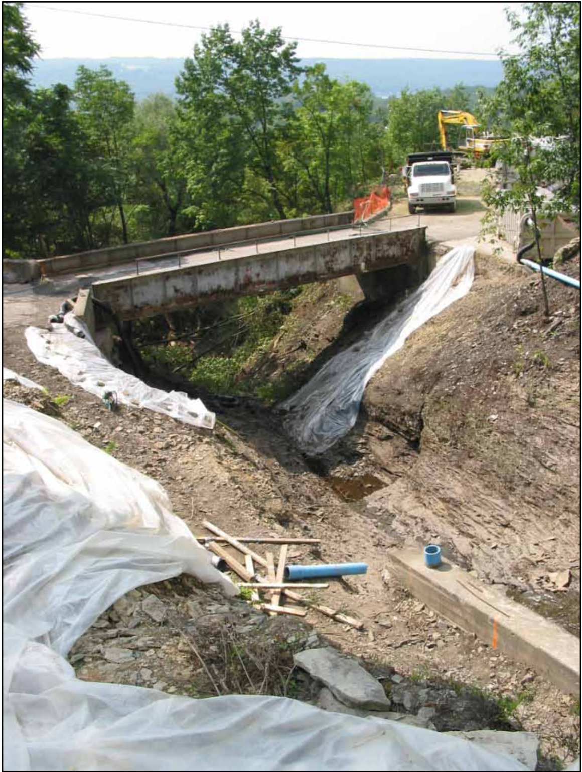
Fig. 56. EPA cleanup of upper raceway before plunge pool. (Photograph by Liska Clemence, 2003, courtesy of Kathryn Gleason).
