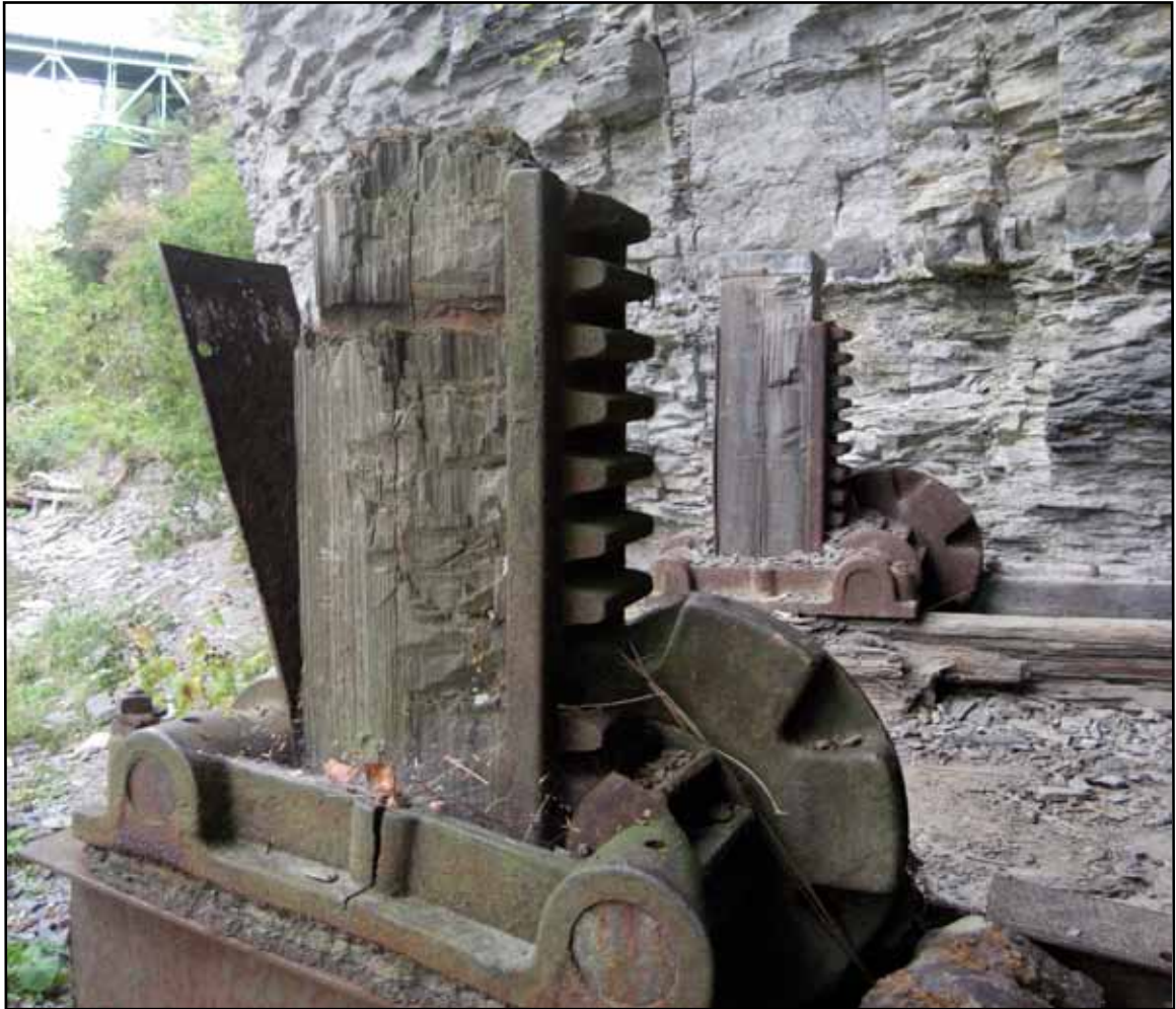
Fig. 101. The hand-operated rack and pinion that lift the gate up and down. (Photograph by author).
