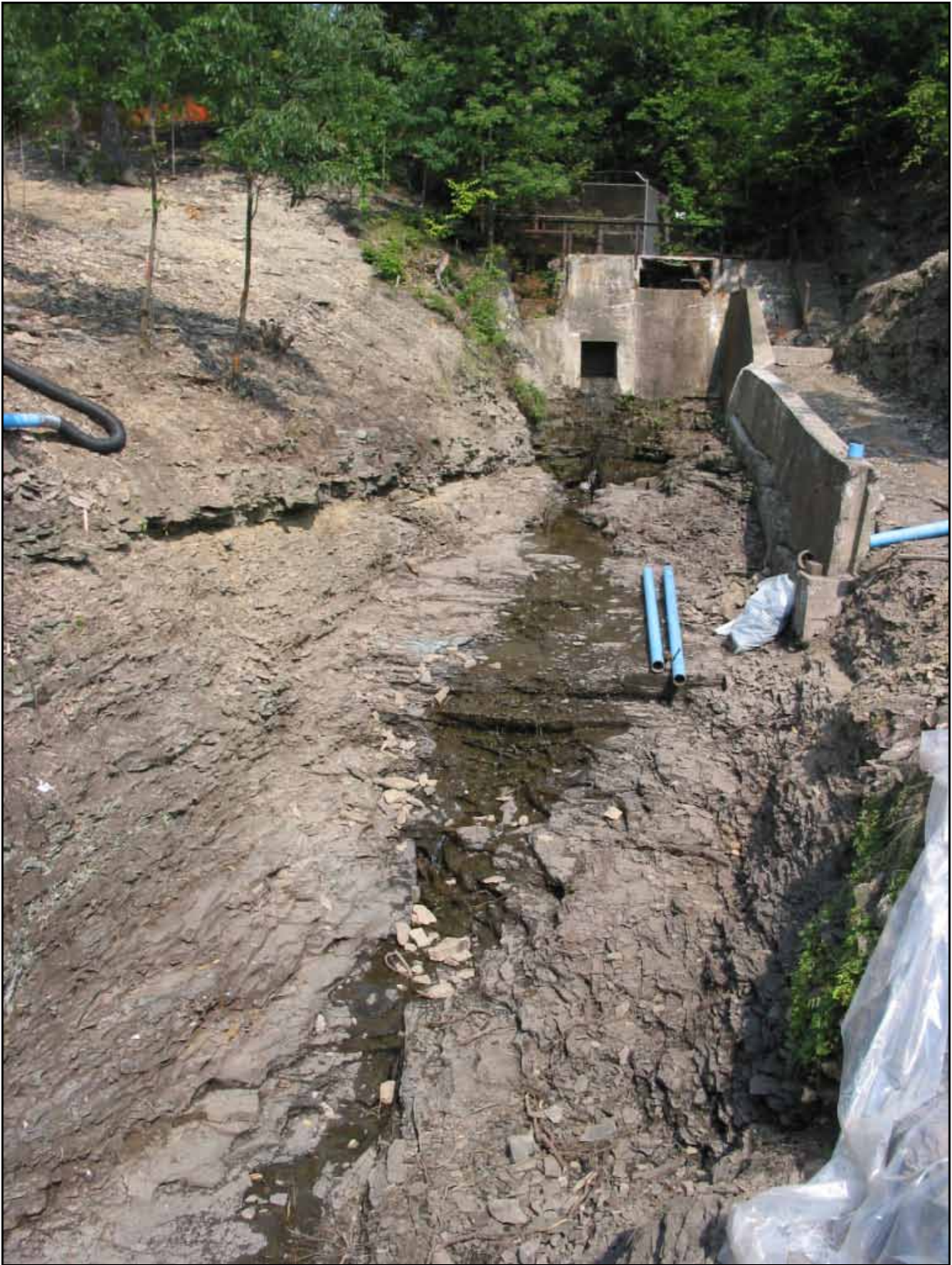
Fig. 55. Cleanup of raceway above bridge. (Photograph by Liska Clemence, 2003, courtesy of Kathryn Gleason).
