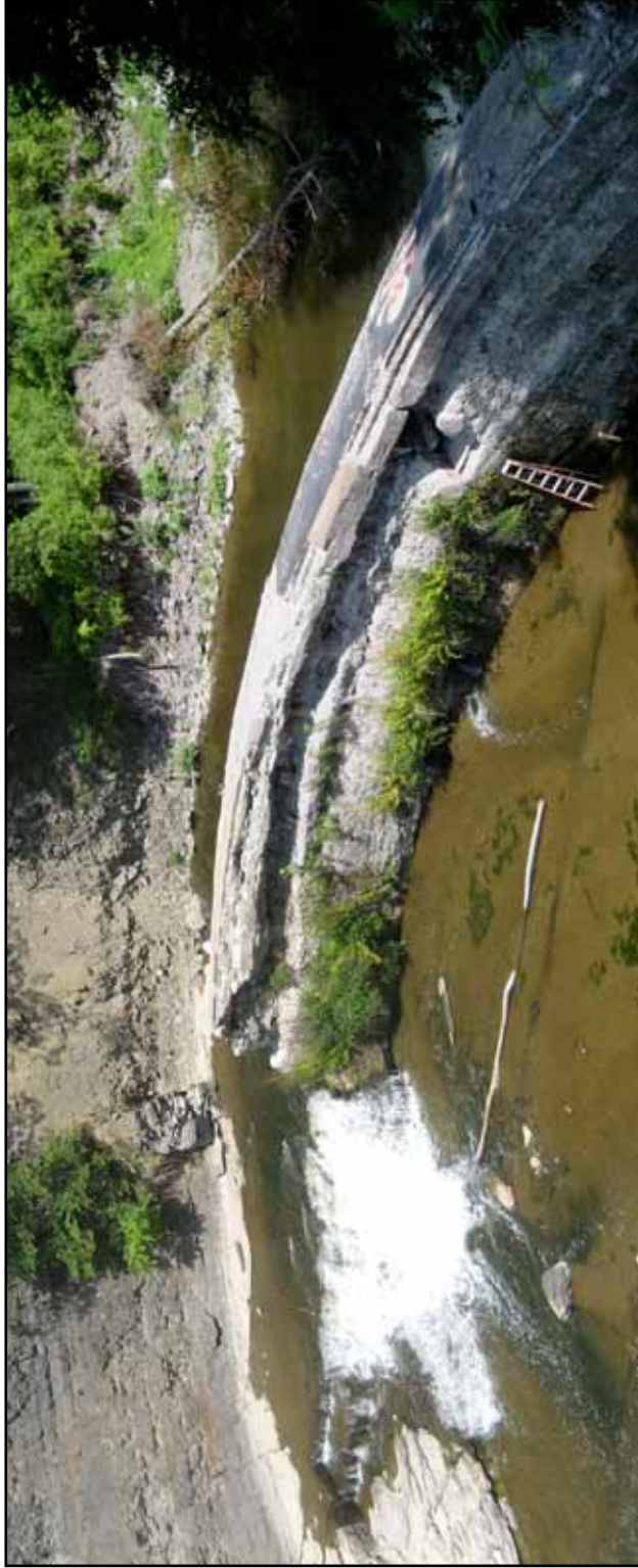
Fig. 98. View of the dam from above. The concrete sill has eroded and the front of the dam is exposed. (Photograph by author).
