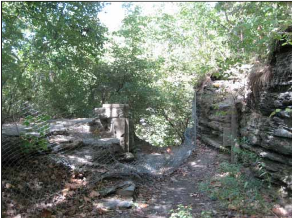
Fig. 116. The terminus of the raceway channel. Water was historically diverted to the left and out of the picture to the flour mill, while the rest spilled over the cliff in the center of the picture and reentered Fall Creek. (Photograph by author).
