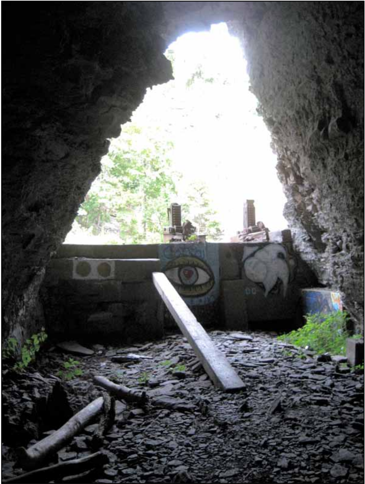
Fig. 102. Profile of the tunnel mouth with the back of the sluice control. (Photograph by author).
