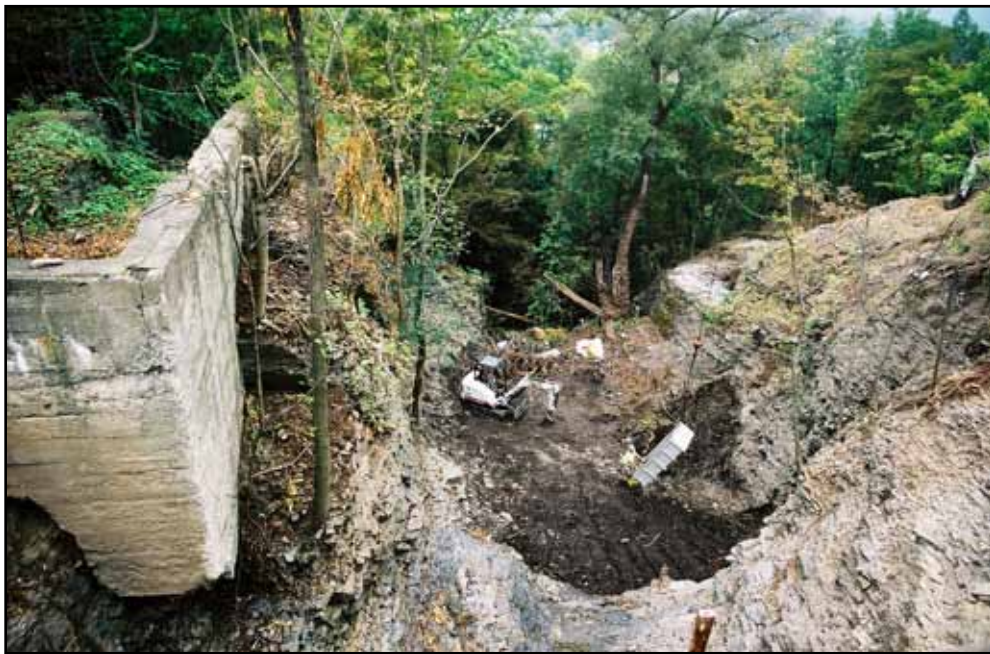
Fig. 44. EPA cleanup of middle raceway below plunge pool with foundation of the original gun company building at left. (Photograph courtesy of Kathryn Gleason, 2004).
