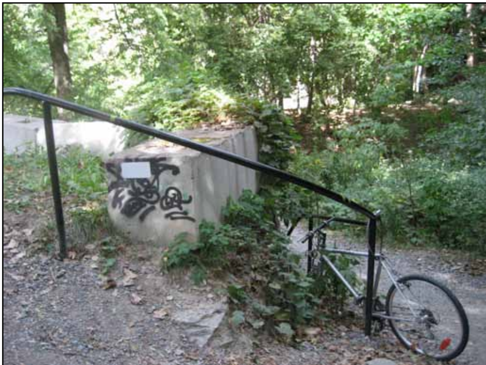
Fig. 75. Staircase leading to the creek's floodplain at the southeast corner of the park entrance. (Photograph by author).
