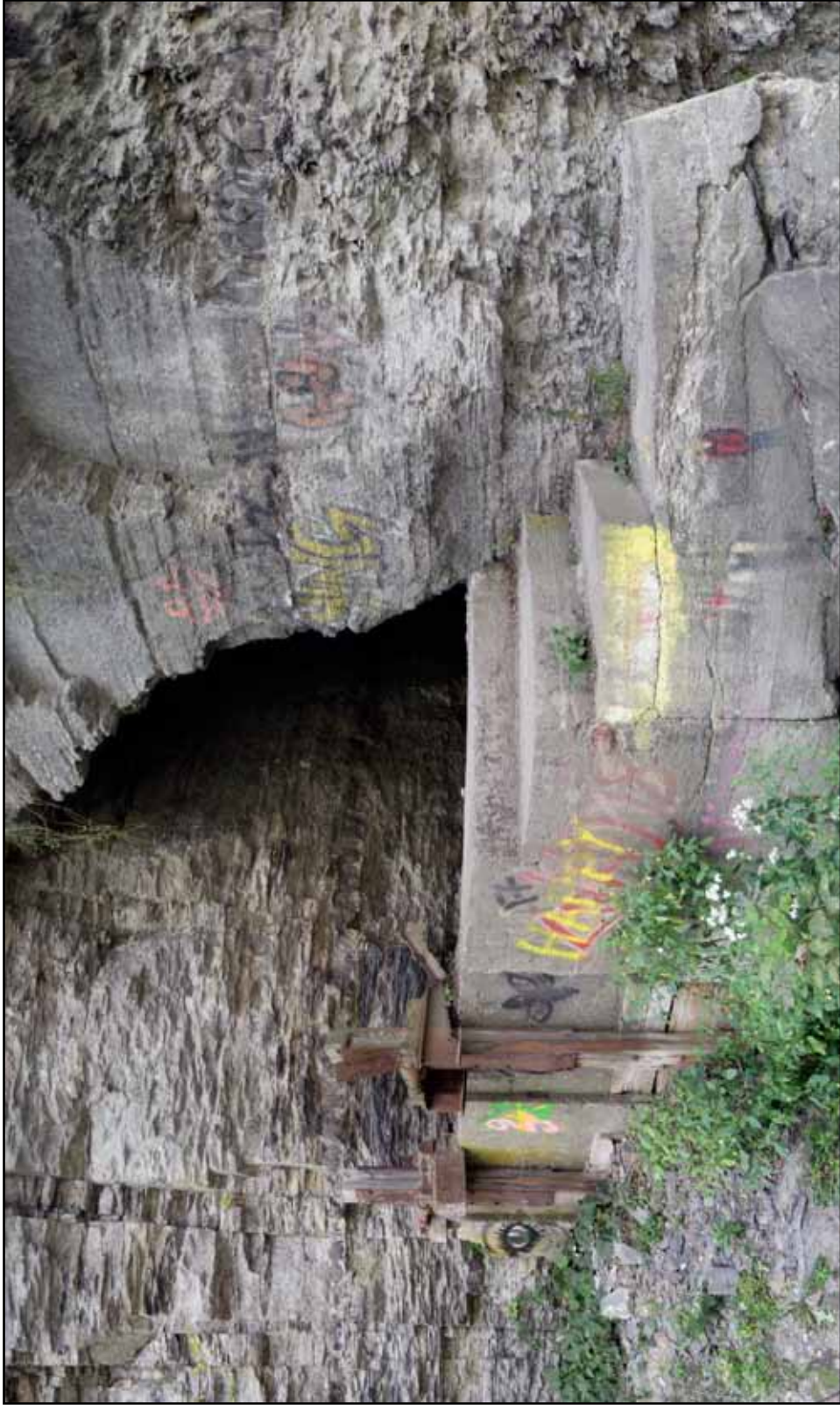
Fig. 100. The sluice gate at the head of the tunnel used to control the flow of water under it and into the raceway. Slag and debris have built up along its base and obscures the wooden gate, which is only partially visible. The staircase leads from the gate to the top of the dam. (Photograph by author).
