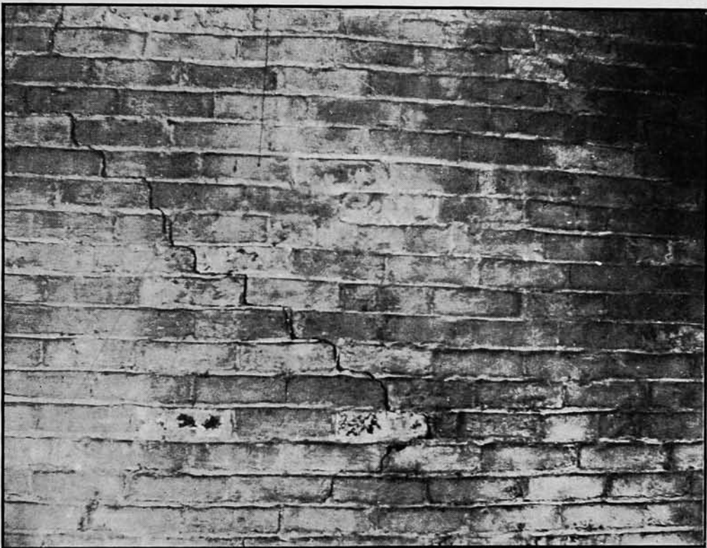
Crack in the South Wall of the Crew Room.
