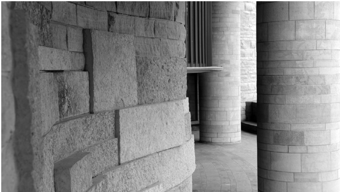
Figure 11: Roughback stonework at the foundation of the museum building, north facade. Photo by Author.
