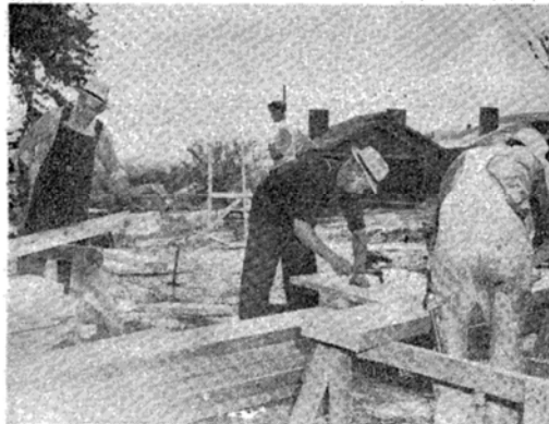
Carpenters were busy yesterday as work was started on the Western Heights project.
