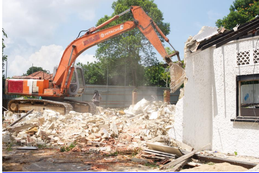
Figure 34: At the close of Villa Alicia, the house, which had been sold to a private developer, was demolished. (Credit: Villa Alicia/Alecia Neo, used with permission.)
