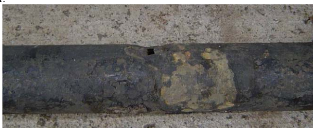
Figure 3. Corrosion of black iron heating pipe.
