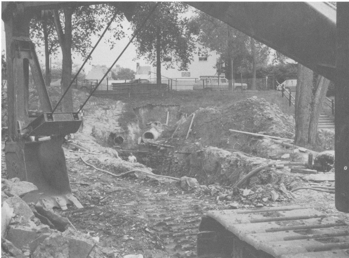
Glen next to Day Hall is torn up during boring of holes for new storm sewer lines (center) under campus's East Avenue.
