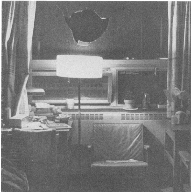
One of more than a dozen bedroom windows broken in Donlon.
