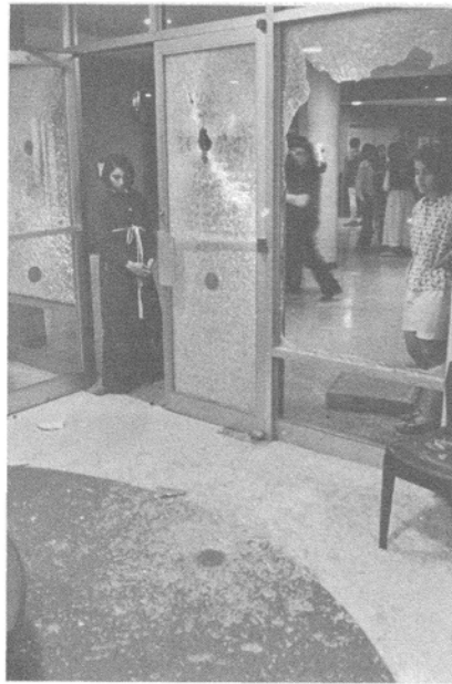
Donlon residents survey damage April 8.
