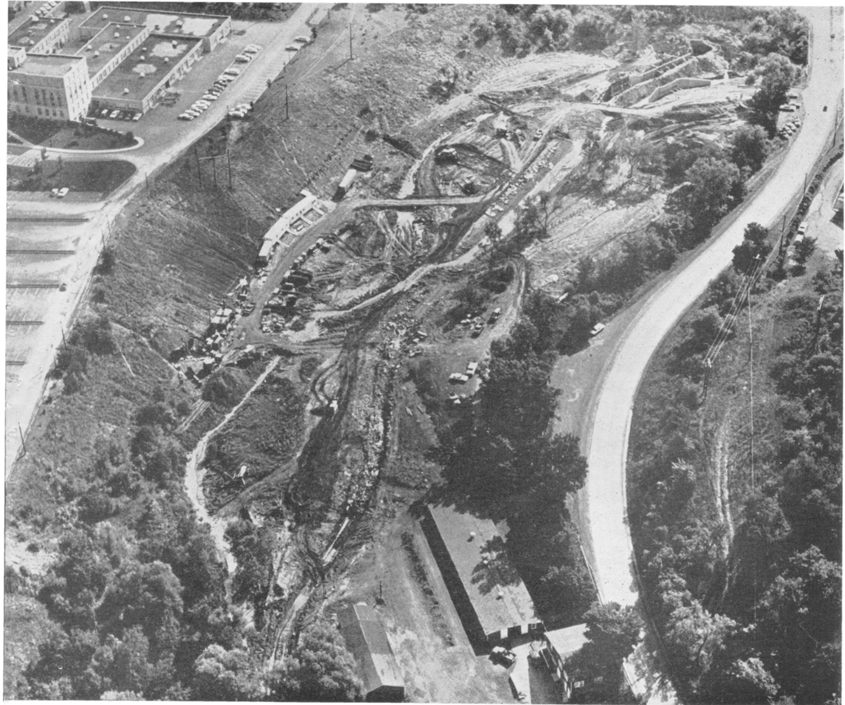
Construction equipment in the bed of Cascadilla Creek where a tunnel 700 feet in diameter is being driven under Upper Alumni Field. Tunnel will house the university's new 10 BEV accelerator for the study of particle physics. Creek-bed is being relocated to make way for laboratory building which will stand at the tunnel head.
