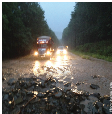
A section of NY-30 in Delaware County washed out during heavy rains
