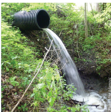
Water discharging from a culvert in Columbia County
