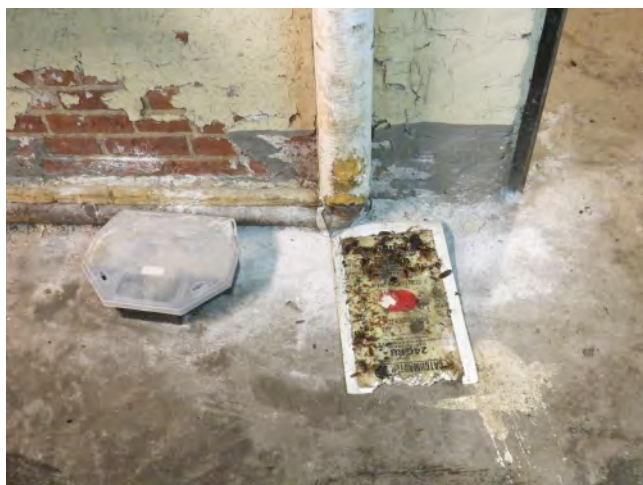
Figure 1. Excessive use/amount of tracking powder as evidenced by clumping; inappropriate placement in an unprotected area: both violations of the label and law.
